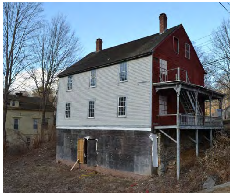
The c.1763 David Greenleaf House located at 2 Town Street ; the rear exterior restoration of the house. Feb. 2020
